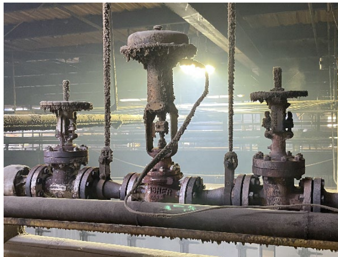
Figure 1 – Original Dryer Steam Control Valve
