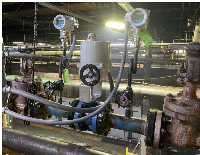
Figure 2 - New Dryer Steam Control Valve & Pressure Transmitters
